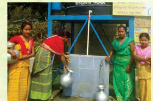
Solar Water Unit for providing safe drinking water installed at Barpeta, Assam
